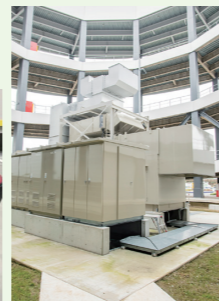
In-house power generation facilities
